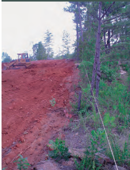
Erosion from construction activities can cause significant damage.
