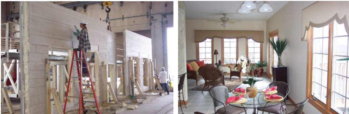
Figure 5. Exterior and interior finishes as part of concrete wall system (a) Simulated masonry during final stages of construction in precast plant (b) Interior concrete wall in residence (Photos courtesy of Dukane Precast, Inc www.dukaneprecast.com )
