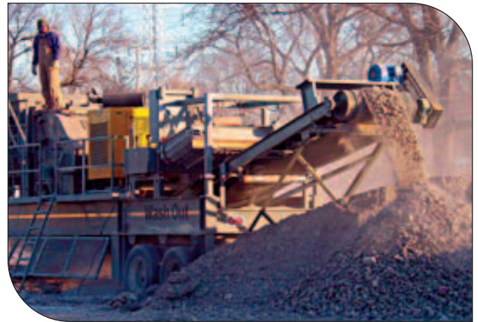
Materials and Resources Credit 2. The picture shows machinery taking portions of concrete walls, columns, and floors and crushing them to be used as fill material.
