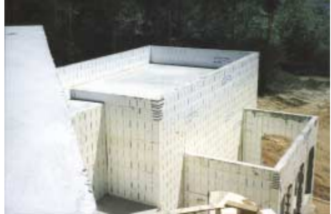
Fig. 2: ICF building with concrete between forms before the exterior finish is applied (Photo courtesy of Polysteel Southeast Distributors)
