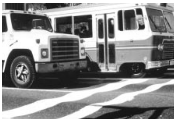
Figure 8. Extreme case of rutting on ACC pavement. (S-56601)
