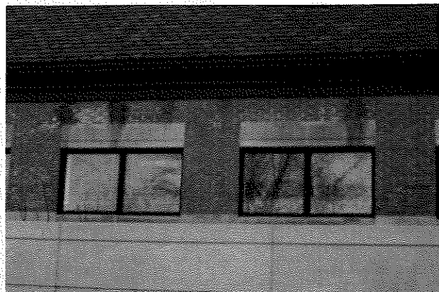
Figure 1 Stains on brick masonry below pool area roof eaves.
