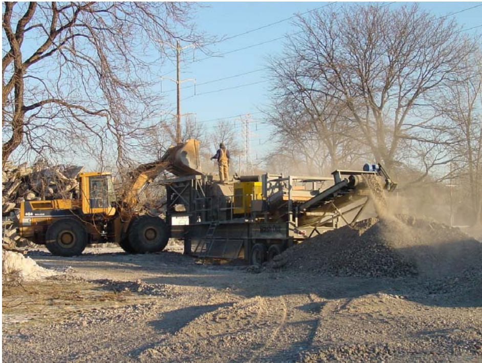
Fig. 3 Demolished concrete being crushed for reuse as fill material on a site
